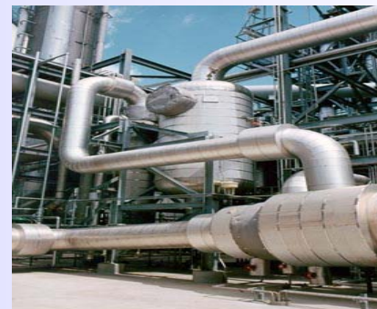
Tail Gas Expander and NOx abatement unit
